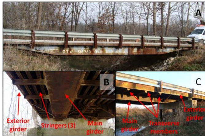
Figure 2. Permanent RRFC Bridge in Indiana Supported at Original Truck Supports (from TR-2-2013)
